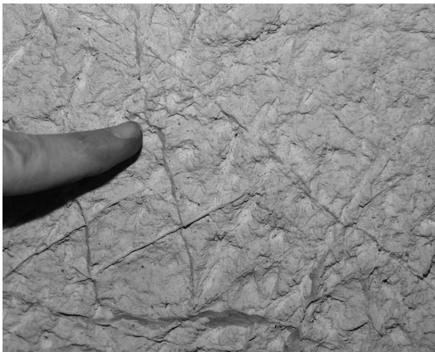
Fig. 5: Outstanding of calcite veins was formed by selective corrosion. Weathered limestone is porous and wet.
